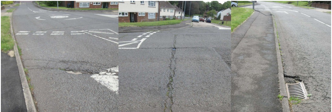
Broken road surfaces above, and below, the roundabout junction of Bishopdown Road and Denison Rise. Below the junction, this drain has sunken hazardously.
