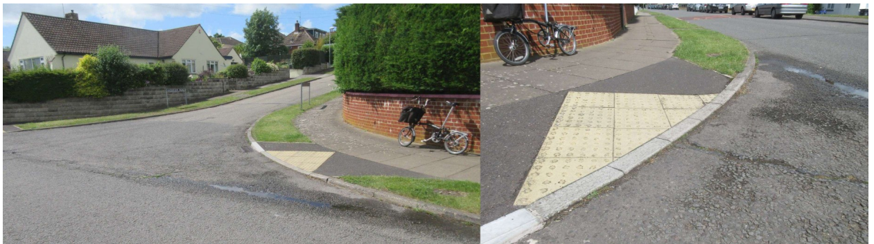
Footway crossing entrance from Bishopdown Road from Anderson Road. The road surface is poor, and the drop kerb is not flush with the road surface.
