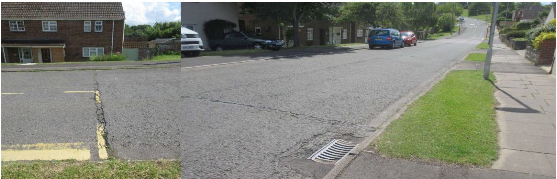
Trench opposite 32 Bishopdown Road. Further down the road a poor Drain Cover.
